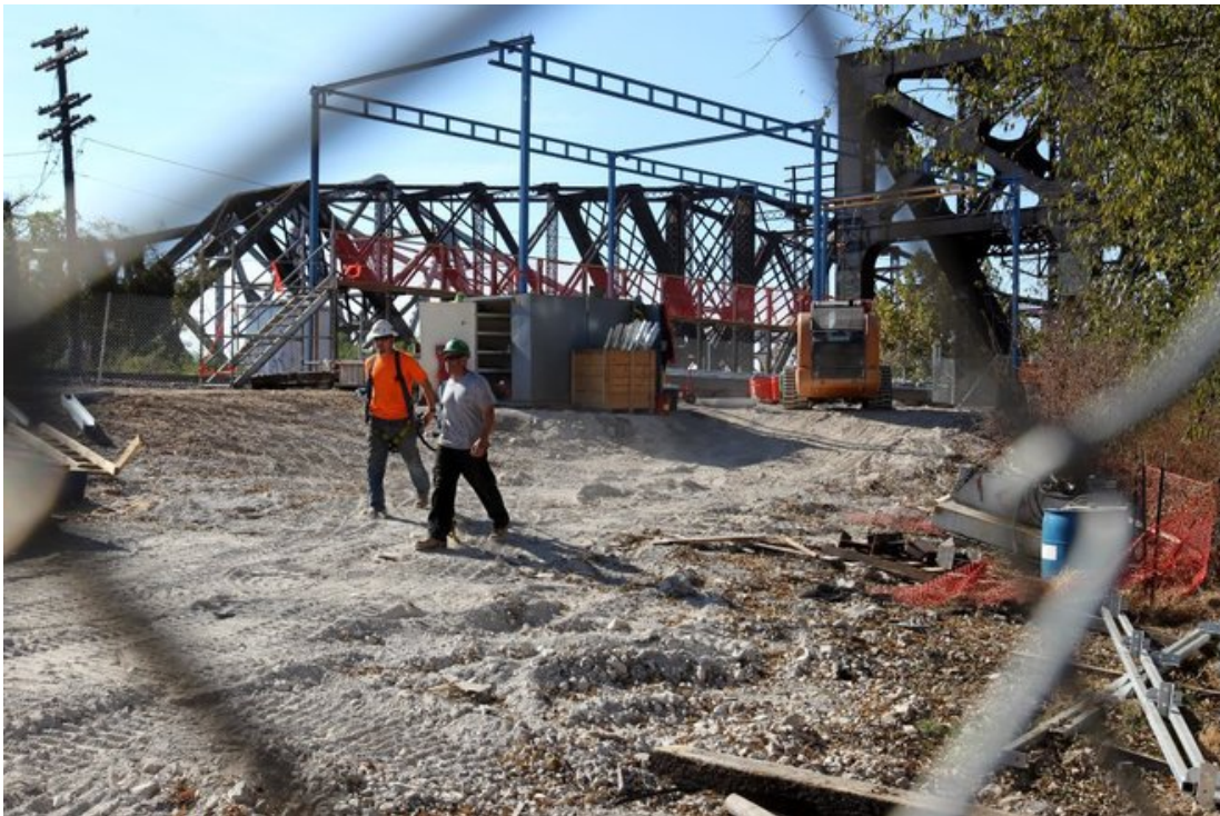
October 22, 2015 - Construction workers leave for the day from working on the Harahan Bridge Boardwalk. The boardwalk has been extended across almost half of the Mississippi river. (Nikki Boertman/The Commercial Appeal)
